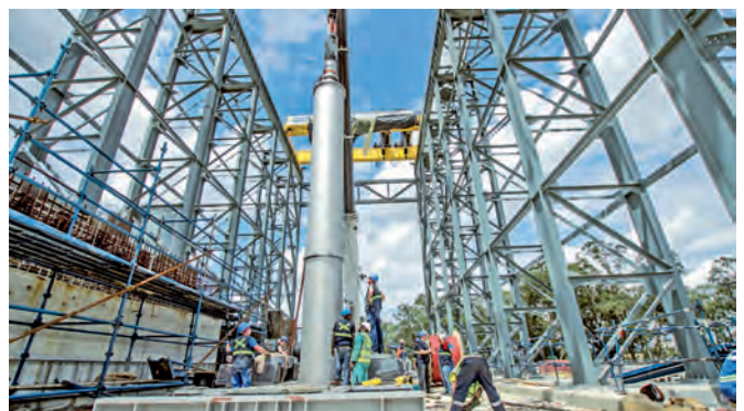
For RAG's German coal mine closure project, ANDRITZ will manufacture and deliver a total of three double-suction submersible motor pumps based on the patented HDM technology
